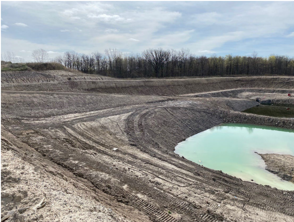
Photo 2- East side wall of Cell 20-1, April 19, 2023.
