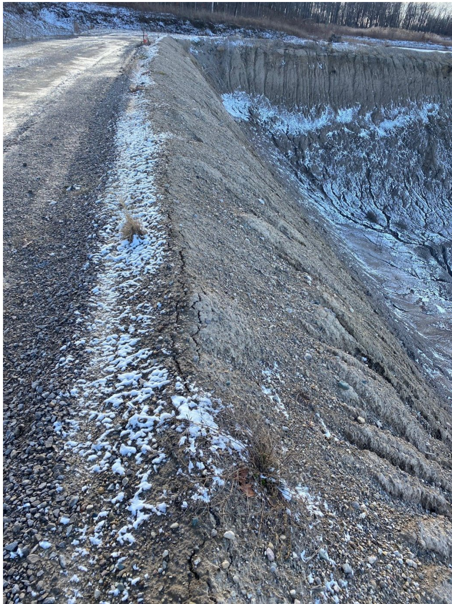
Photo 20- Cell 20-1 East side wall, looking south. Note minor cracking along the top of the slope, due to surficial sloughing, December 19, 2023
