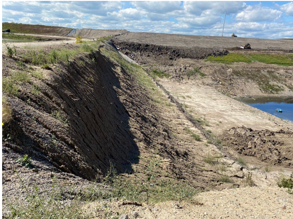
Photo 14- South side wall, looking west. Side wall sloughing, but stable, September 14, 2023.
