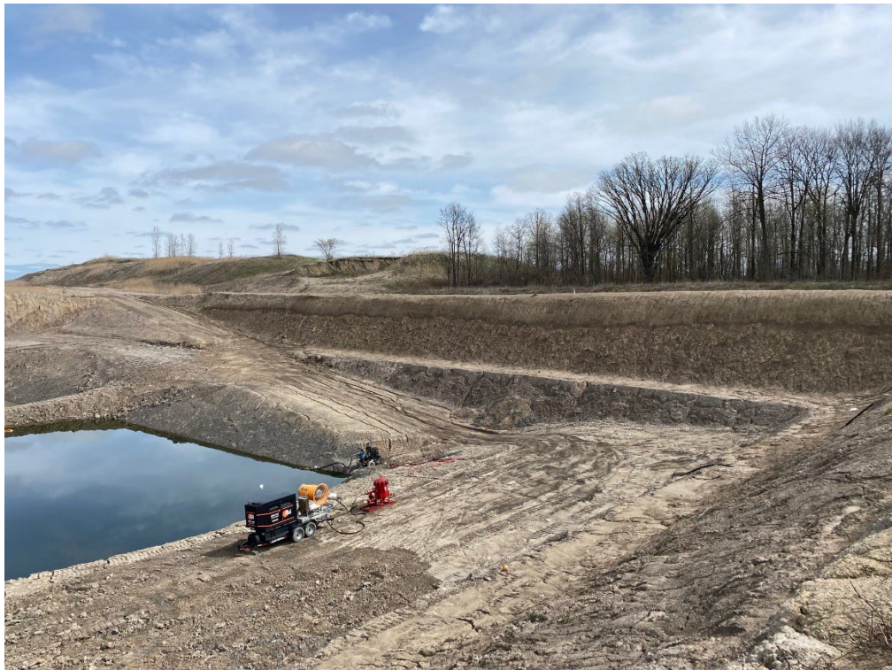
Photo 6- Cell 20-1, East side wall, April 19, 2023.
